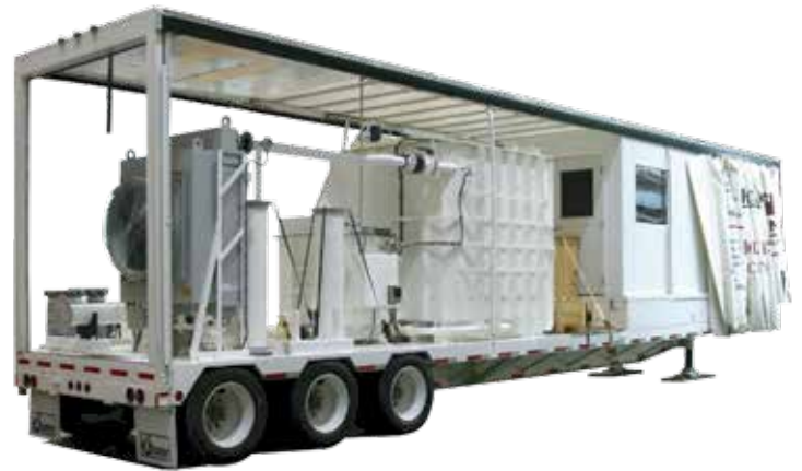
Variable Frequency, 265 kV, 22 MVA
