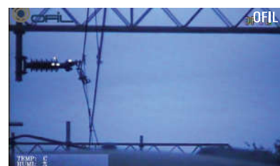
OH catenary Corona insulator
