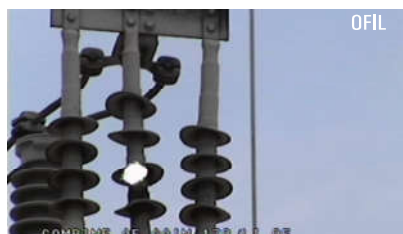
In substation Corona on terminator
