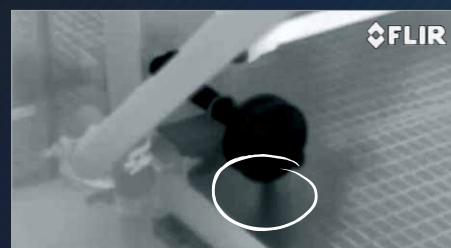
LEAK IS CLEARLY VISIBLE ON THE THERMAL IMAGE
