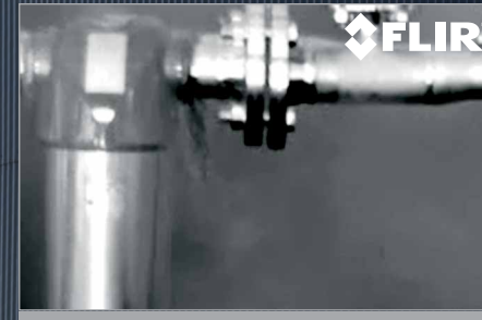
SPOT HARD-TO-FIND CO 2 LEAKS
