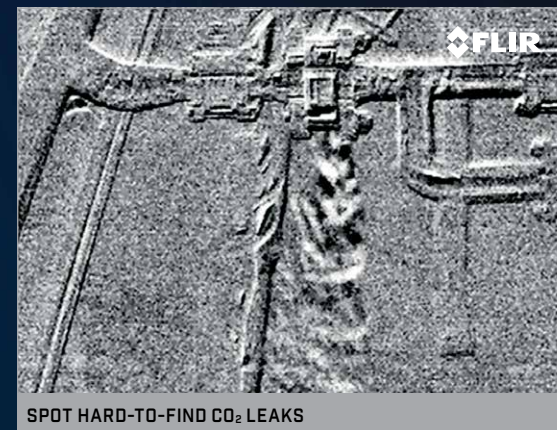
SPOT HARD-TO-FIND CO 2 LEAKS
