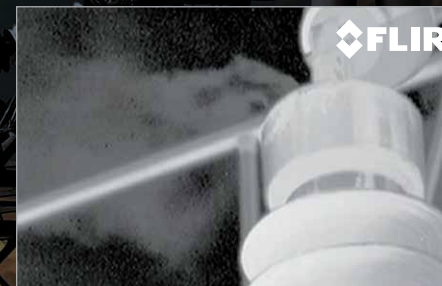
SF 6 LEAKING FROM CIRCUIT BREAKER
