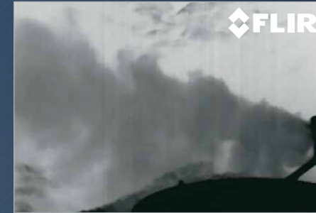
VENTING STORAGE TANK PRESSURE RELIEF VALVE
