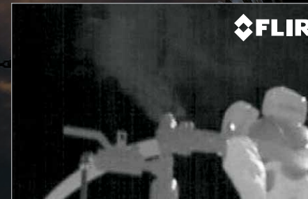
COMMON SF 6 PLUMBING LEAK
