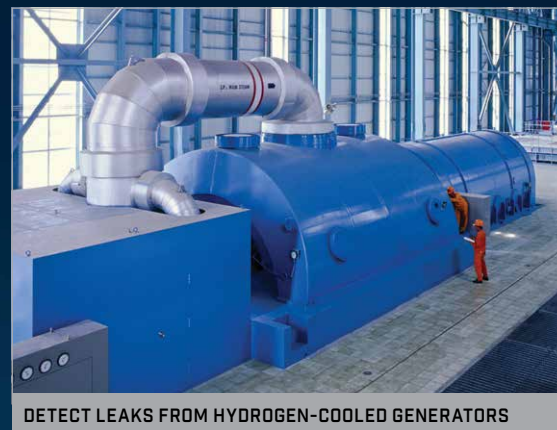
DETECT LEAKS FROM HYDROGEN-COOLED GENERATORS
