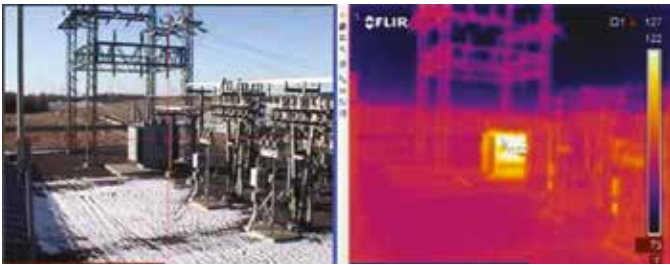
Digital photo and thermal image of a substation showing a transformer with excessive temperature.
